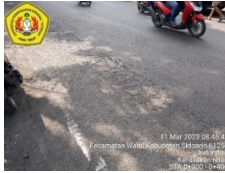
Figure 3. Examples of Crack Damage at Research Locations (Observation Results)
