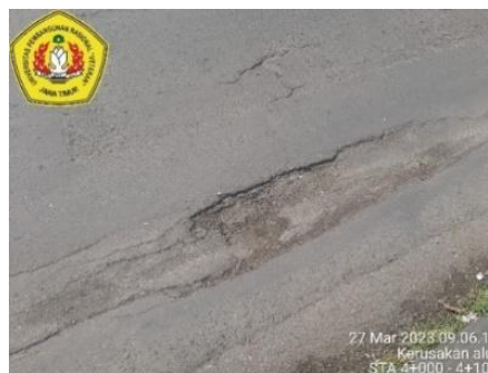
Figure 2. Examples of Flow Damage at Research Locations (Observation Results)
