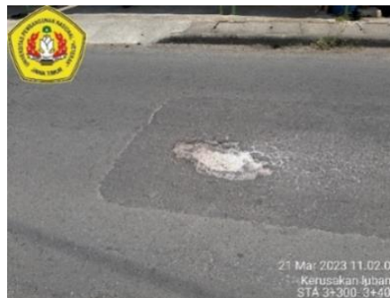
Figure 1. Examples of Whole Damage at Research Locations (Observation Results)
